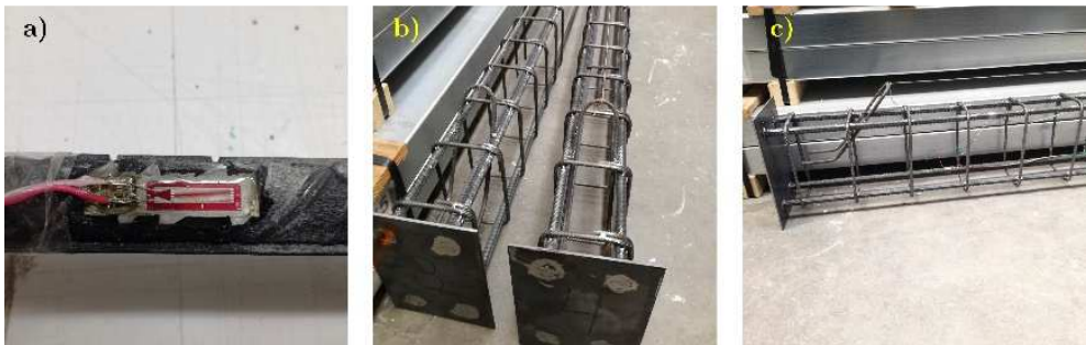
Figure 6.2. Left: Strain gauge attached to the longitudinal reinforcement. Center: Beam reinforcement of V3 and V4. Right: Steel handle for lifting.
